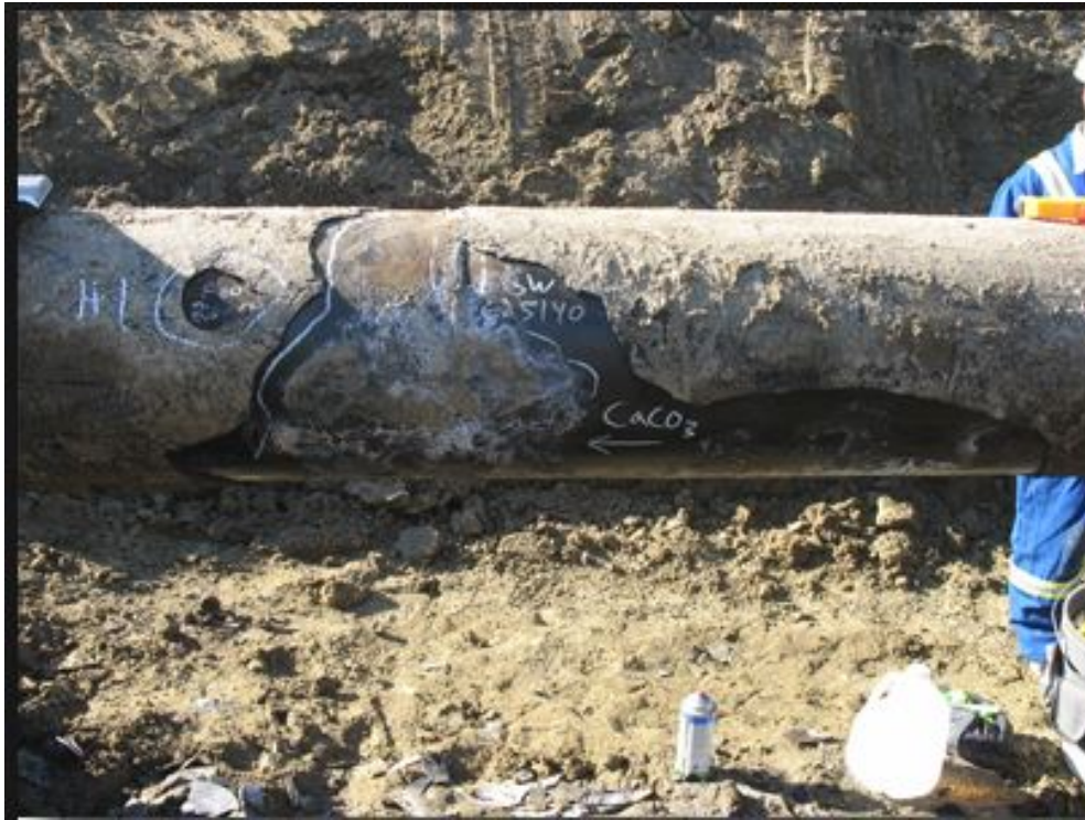
Failure due to stress corrosion
